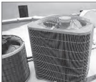
Air conditioning systems
